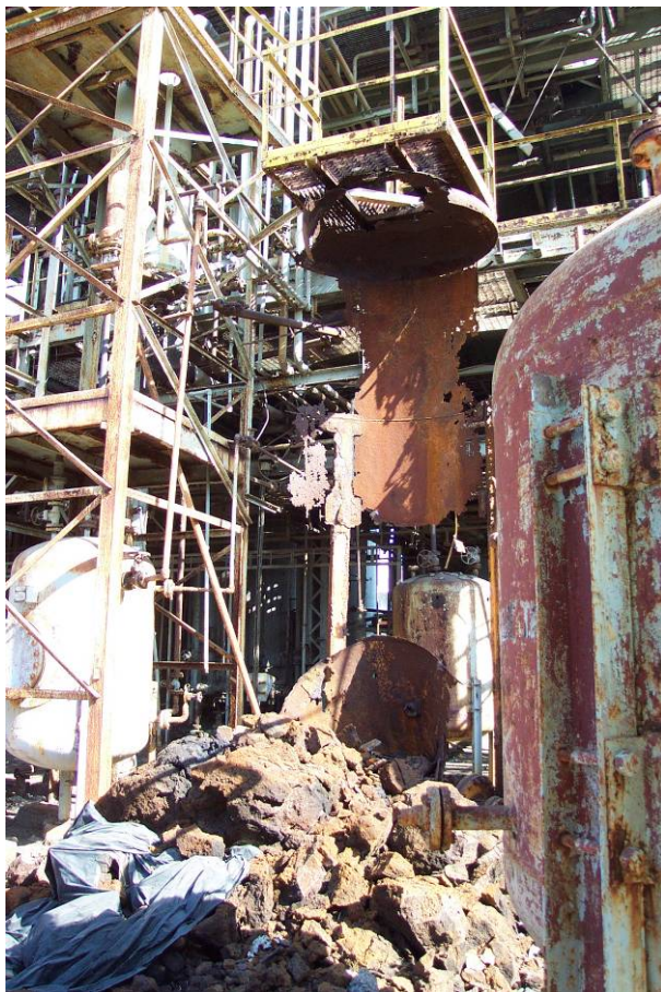
Fig. 14. Corroded tank with unknown contents lying below.
