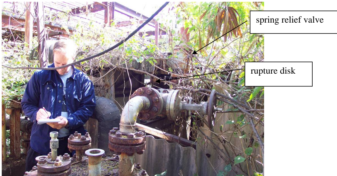
Fig. 9. Photograph of Tank 611 entry piping. Rupture disk is in center, spring relief valve is behind flora that has grown in over the years.
