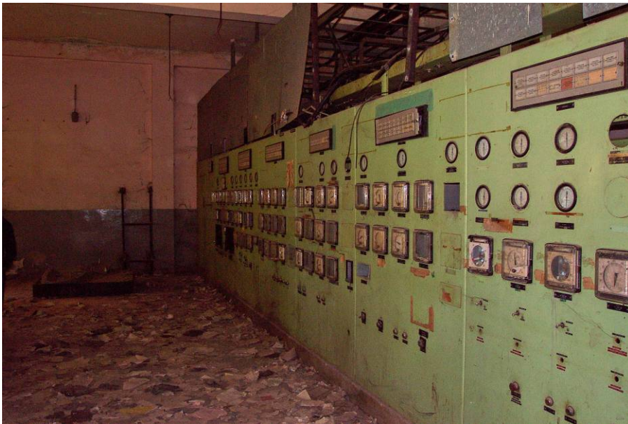
Fig. 12. Photograph of the control room 20 years later.
